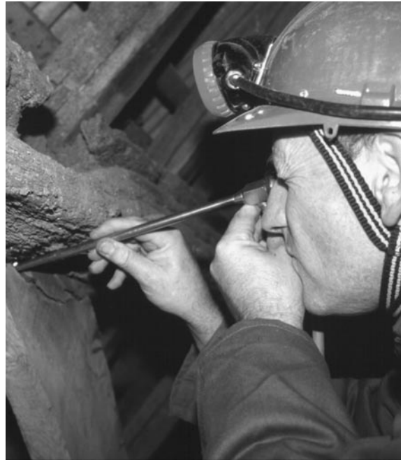
Bat worker using fiberscope to inspect mortice joints in barn. © Shirley Thompson
